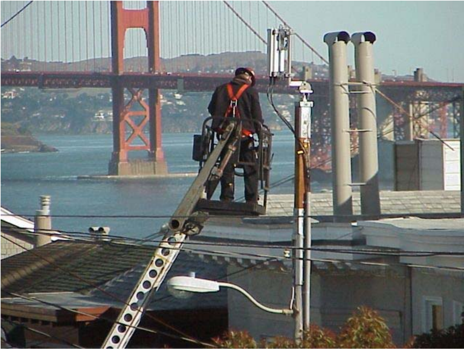
Exhibit 13: A view from a neighbor's house during installation work (taken after filing of the appeal)
