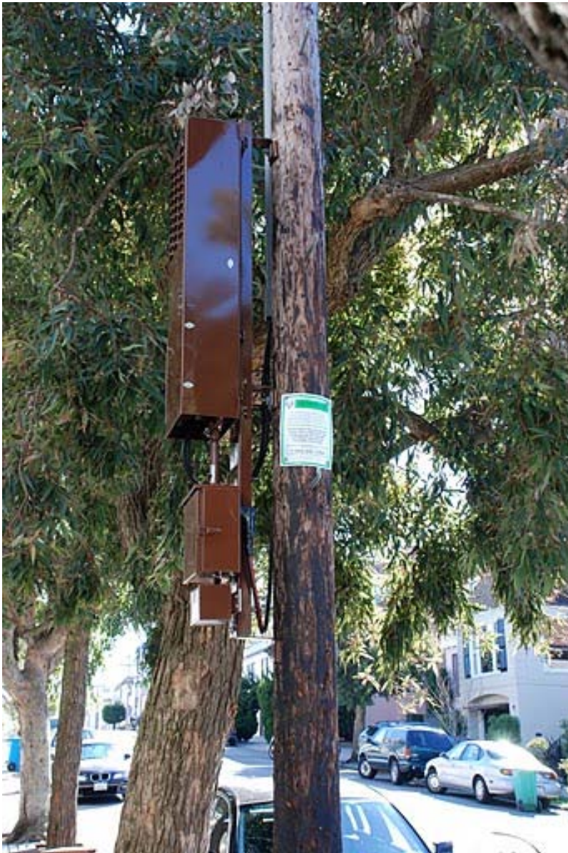
Supporting equipment at 156 27 th Ave
