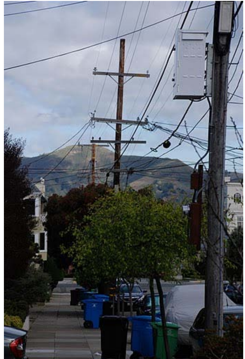
Supporting equipment at 161 27 th Ave
